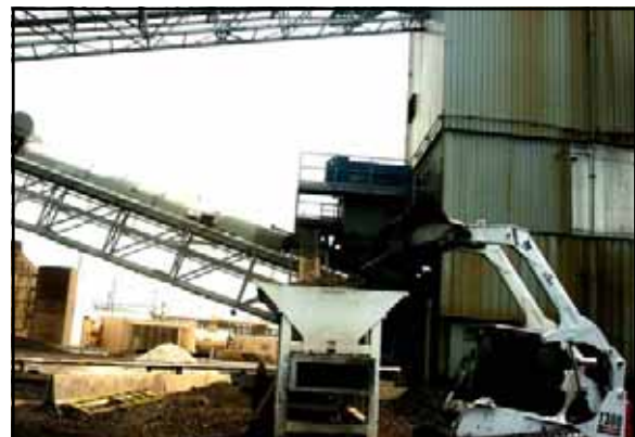
TDF going to the boiler
